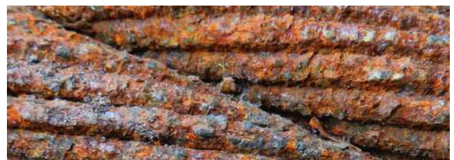
Enlargement of external corrosion
